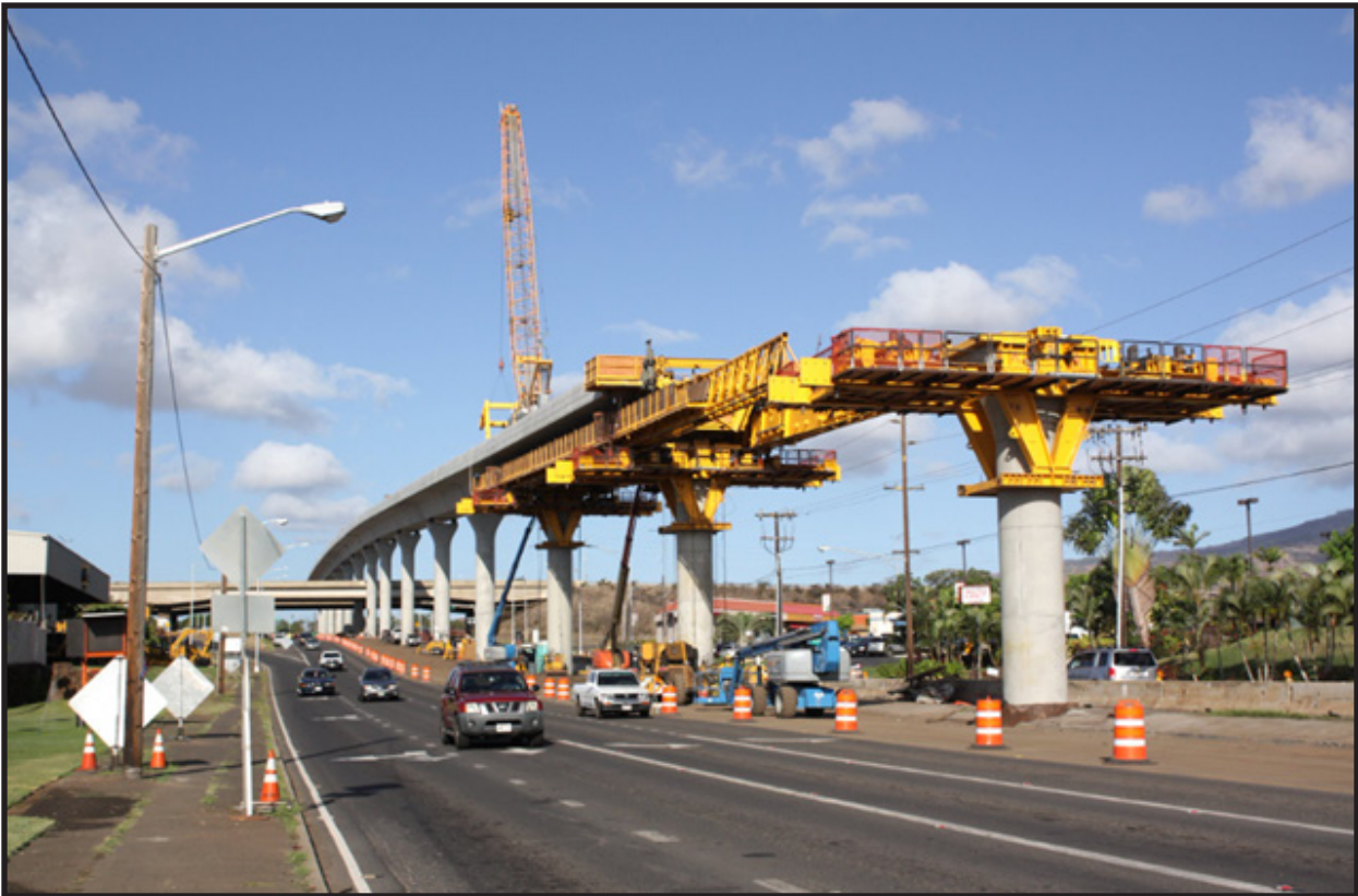
Hawaii's rail project is $5 billion over budget and more than eleven years behind schedule.
